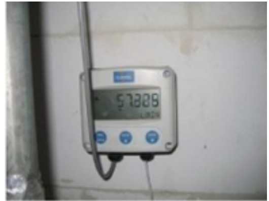
Sprinkler flow-rate meter
