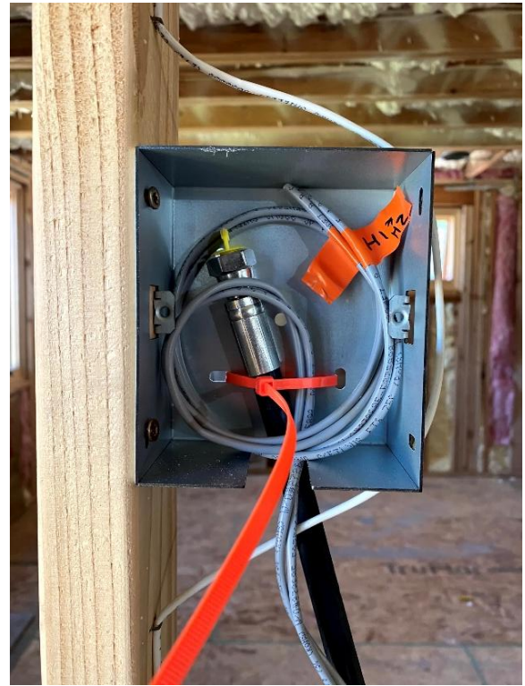
Figure 8 slack for ease of connection data cables
