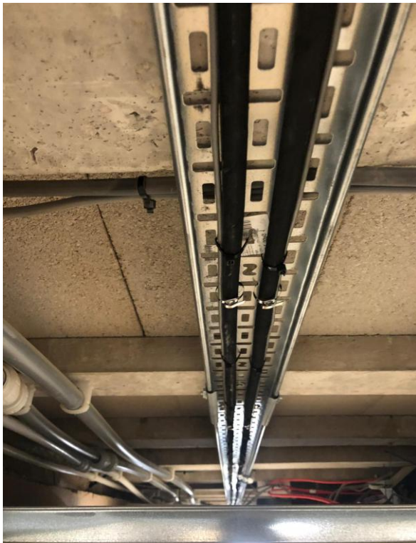
Figure 5 Cable tray hose installation
